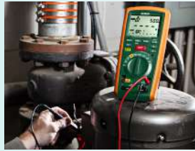
Insulation test on pump motor
